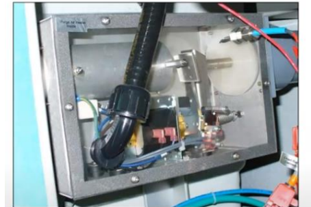
Purge Air Box
