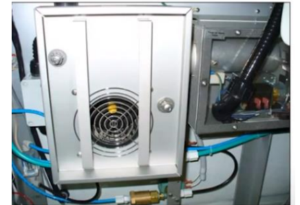
Purge Air Blower
